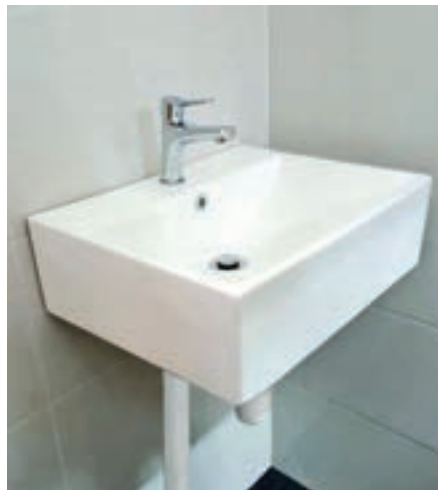
Wash basin with tap mixer
